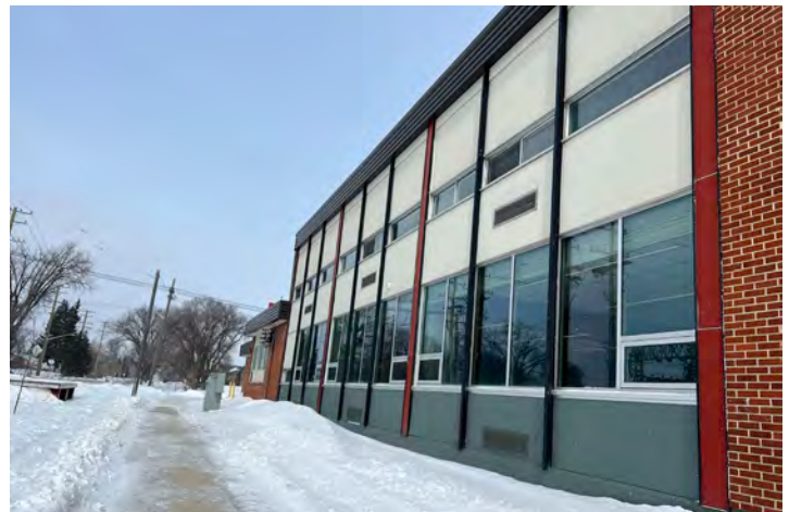
West facing facade, along Speers Rd. after Student Commons renovation where the existing short windows were replaced with larger windows on the main floor.
